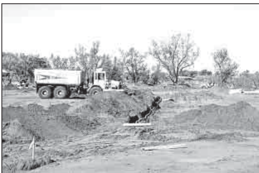
Civil works are well underway for the additional 156 rooms at Camp 3 in Roxby Downs, with the installation of the rooms set to begin later this month and, all going well, completed and handed over in mid-August.
